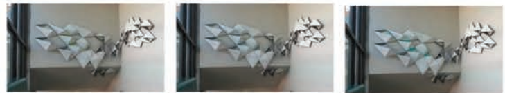
Above and right: The four hour installation process was facilitated by the use of lightweight, preassembled parts.
